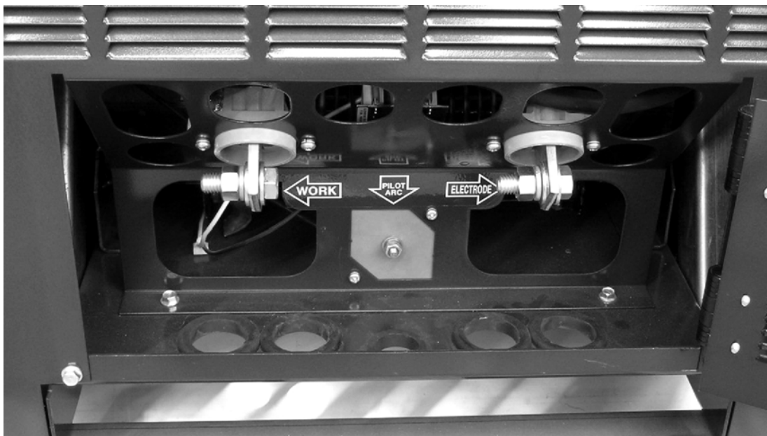
Front access panel opened
